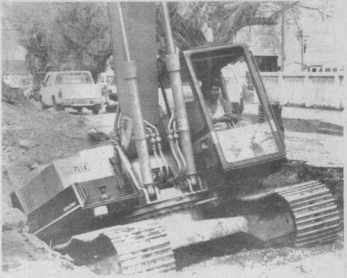
Traffic in Apia yesterday was backed up right through town because of work being done on Mulivai Bridge. According to reports from the site, this will be a common occurrence for another week.
